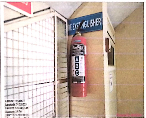
Fire Extinguisher in passage
