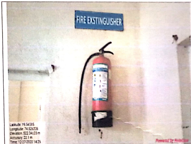
Fire Extinguisher in office
